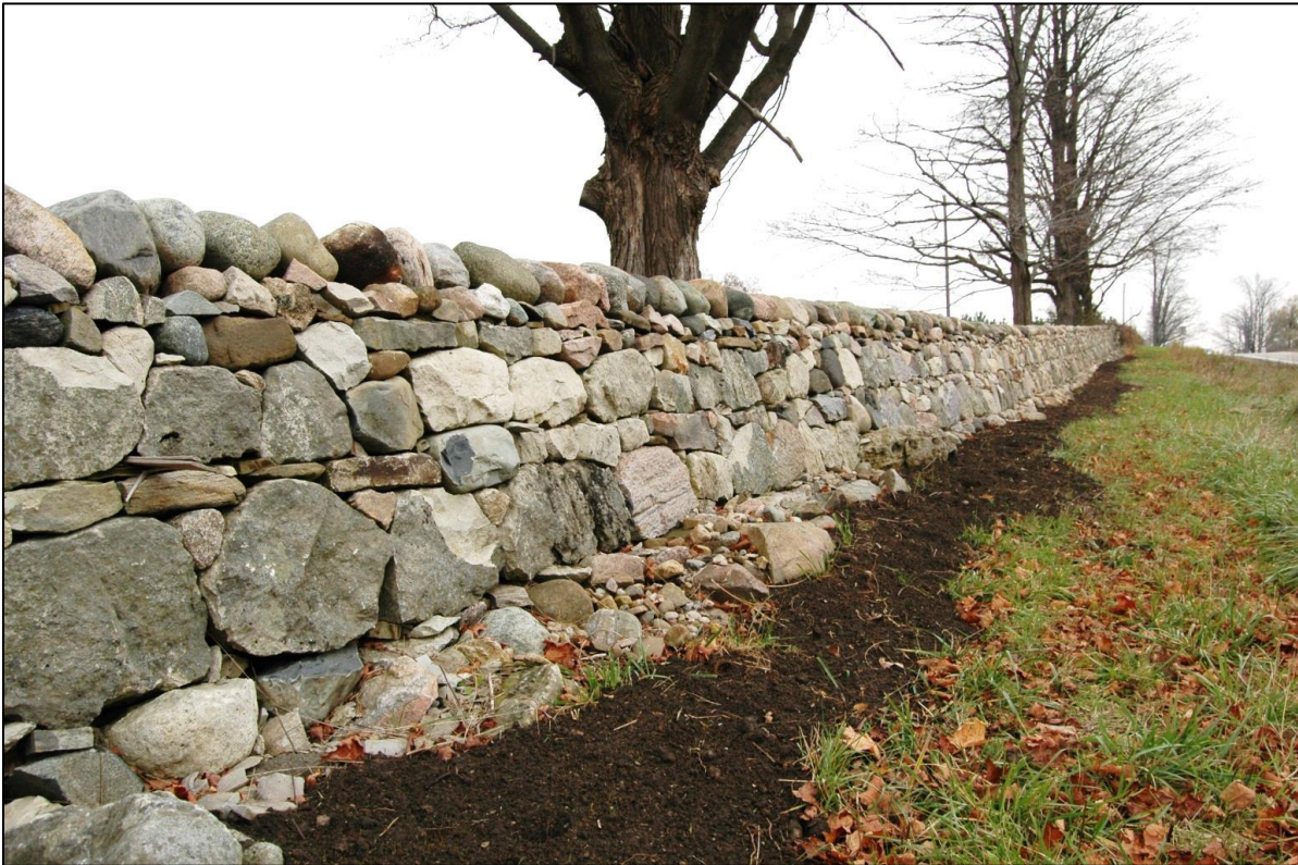
Patullo-McDiarmid Dry Stone Wall: Restored using existing stone and new cedar shakes.
