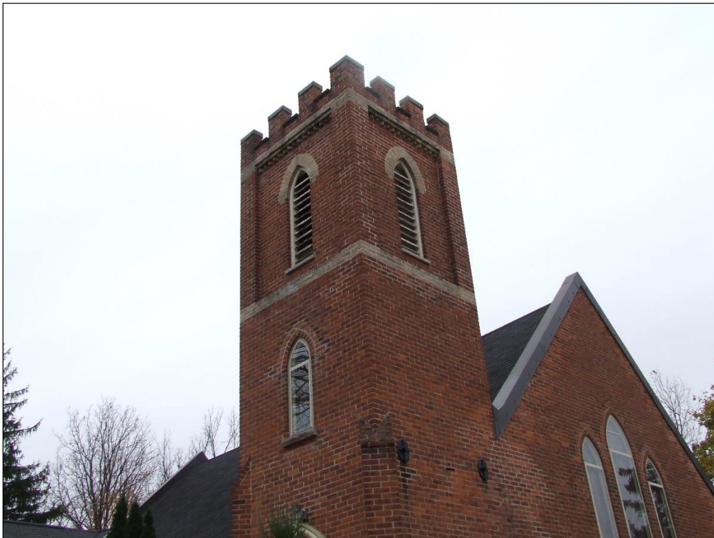
Image 8: Bolton Heritage Conservation District: repointed areas of Christ Church Anglican bell tower
