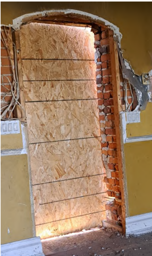
Figure 12: Interior view of doorway on rear (west) façade showing the three wythes brick wall construction, October 2023.
