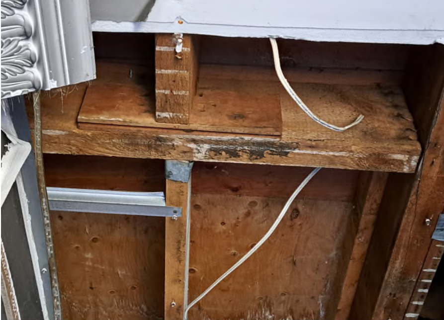
Figure 11: Interior view of large dimensional lumber visible exposed in first floor ceiling near the main entrance to the Thompson-Scott House, October 2023.
