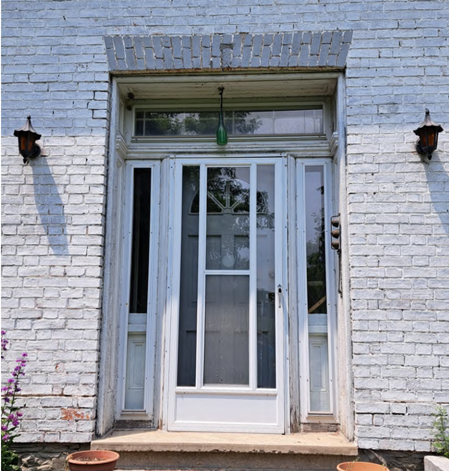
Figure 13: Detail of front centre doorway, including sidelights, transom with tracery and molded wood jamb, June 2023. Note concrete sill.
