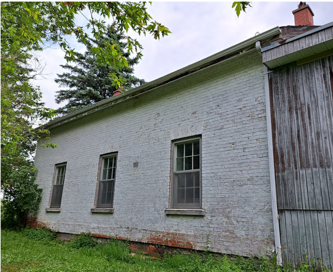
Figure 8: Rear (north) façade of the Robinson Farmhouse, showing original multipane windows, June 2023.
