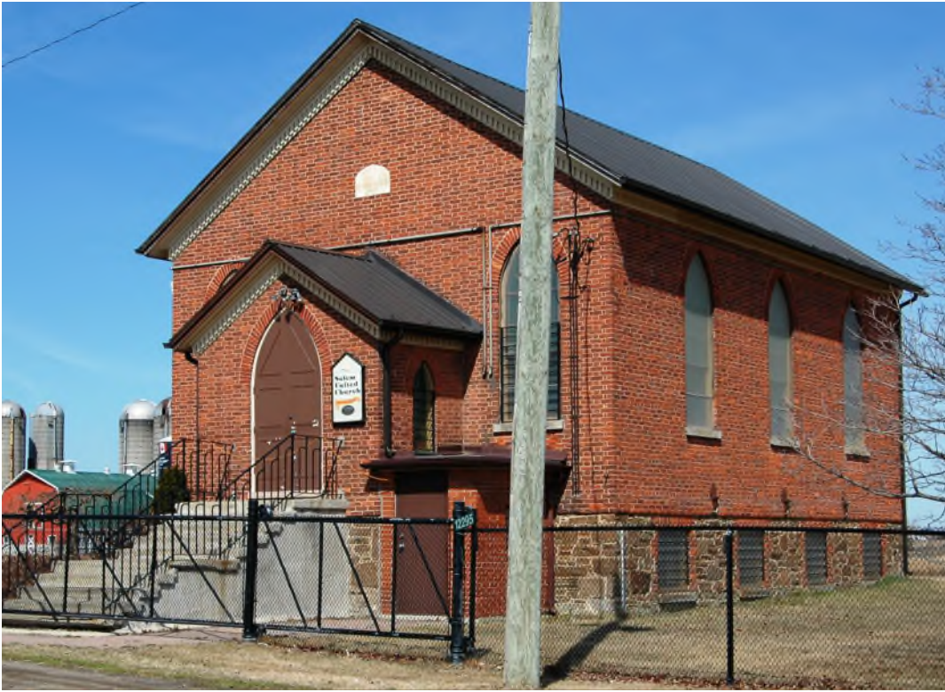
Figure 23: Salem United Church at 12295 Innis Lake Road, its foundation showing the same narrow stone used at 12542 Airport Road and 12620 Airport Road, 2012.
