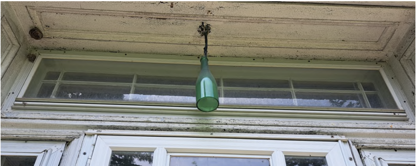
Figure 14: Detail of transom above the centred front entrance showing extant tracery protected by an aluminum storm window, June 2023.
