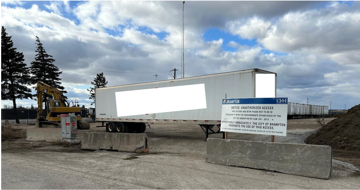
19 Work performed on City Right-of-way to create truck entrance (no permit)
