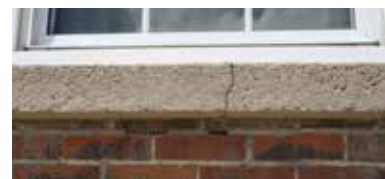
Cracked window sill on east wall (ERA, 2018).
