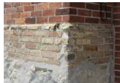
Brick deterioration on the east side of original portion of the building (ERA, 2018).
